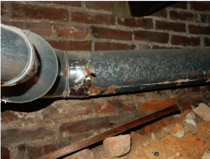
Boiler flue pipe in poor condition. Rusted through, this is a hazard, could lead to CO intrusion. Have licensed contractor replace flue pipe. Remove dirt in contact with flue pipe.
