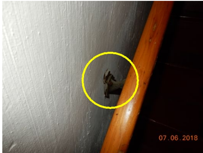
Bracket loose at basement stairs
