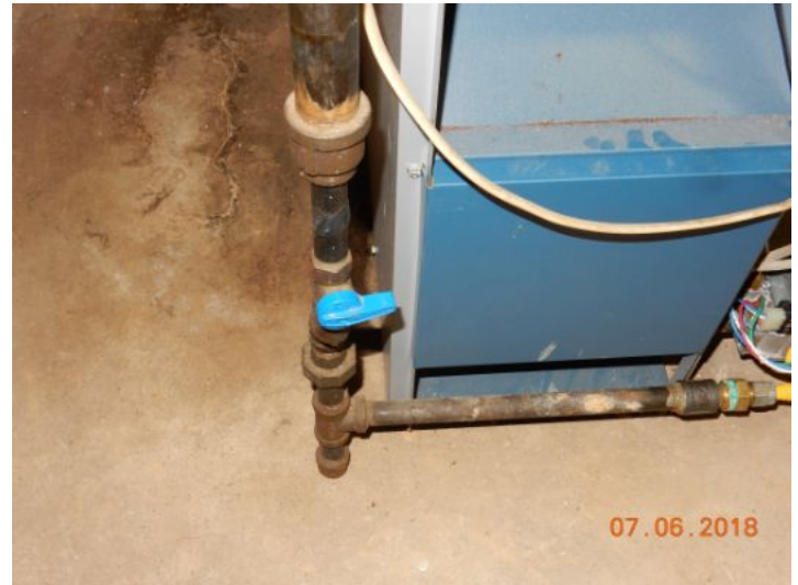
Boiler gas valve was shut off at time of inspection. Could not test boiler. Have sellers activate boiler and have licensed boiler tech evaluate/inspect.
