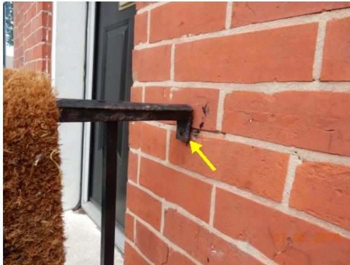
Loose/detached handrailing at front. Secure as necessary.
