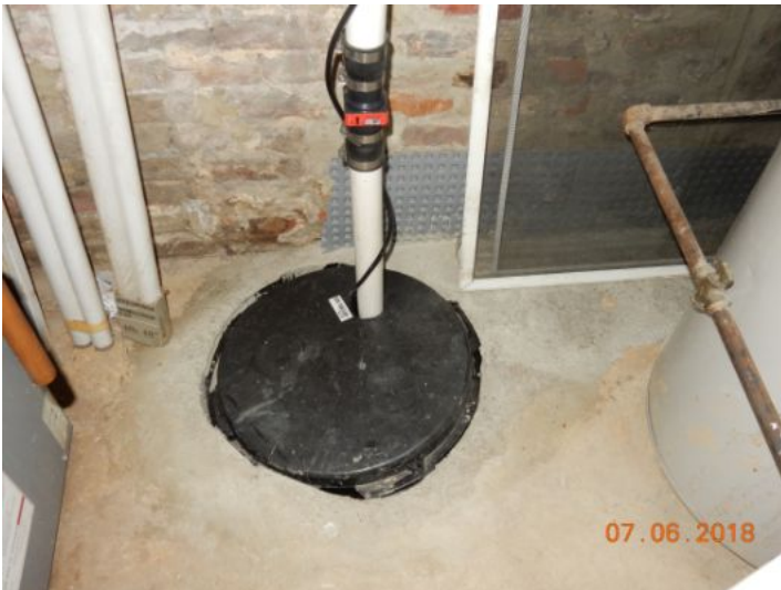
Sump pump operational
