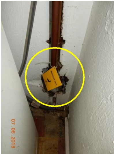
Main water valve location
