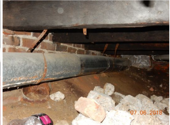
Crawlspace vapor barrier is missing. Recommend installing 6 mil polyethylene over dirt.
