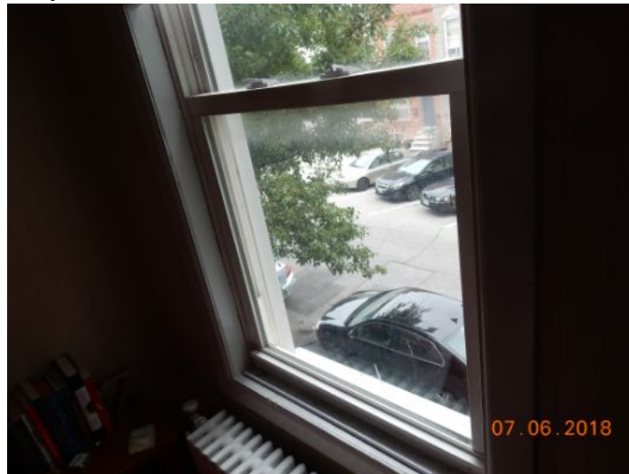
Most window screens missing. Check with seller.
