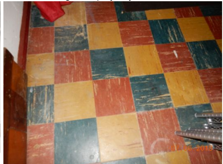
Linoleum tiles may contain some asbestos.
