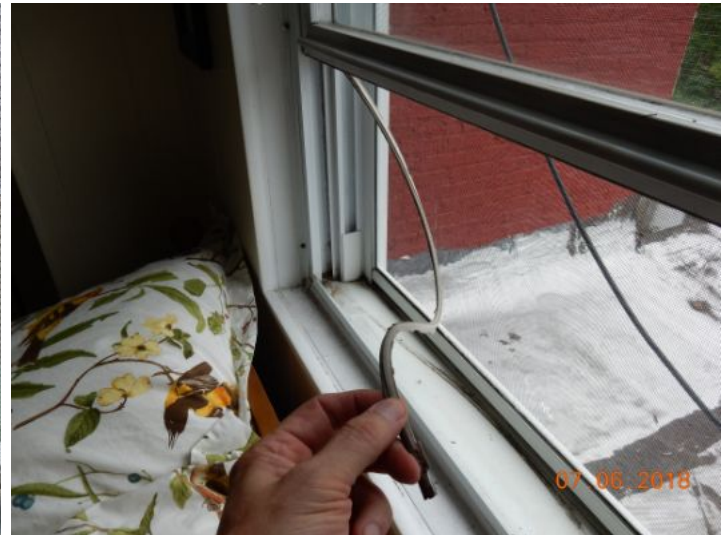
Detached weather stripping
