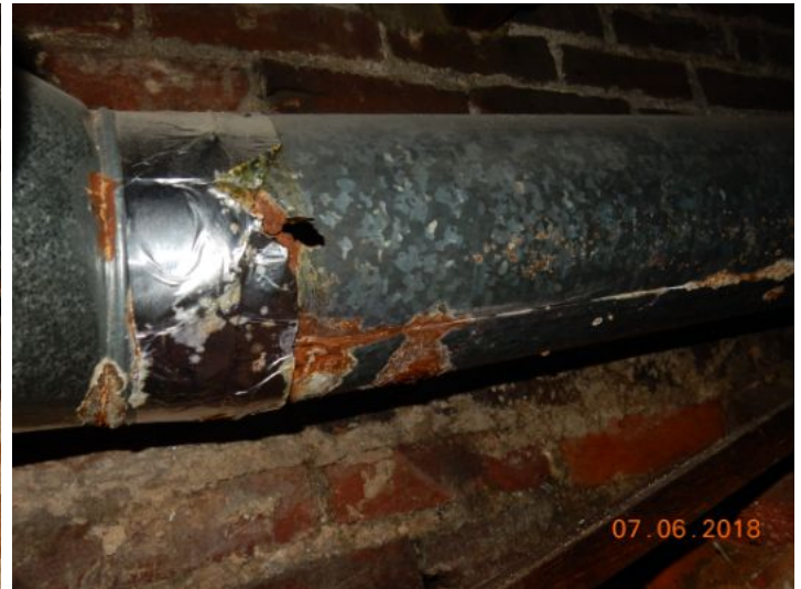
Boiler flue pipe in poor condition. Rusted through, this is a hazard, could lead to CO intrusion. Have licensed contractor replace flue pipe. Remove dirt in contact with flue pipe.
