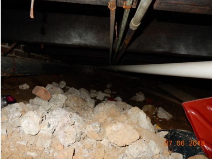
Recommend removing debris from crawlspace.
