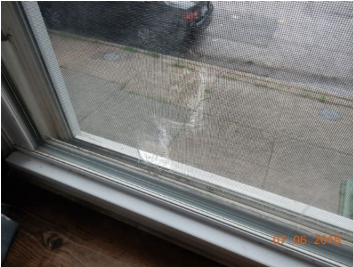
Window screen(s) damaged. Repair as necessary.
