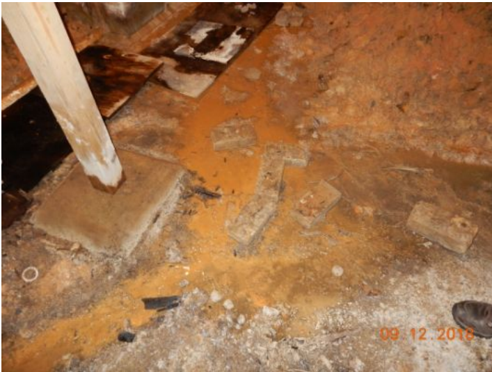
Water pooling in basement
