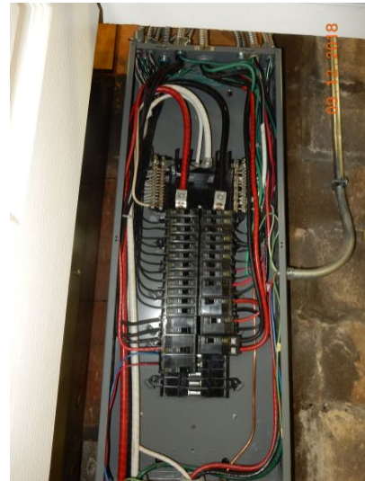
Electrical panel, main office
