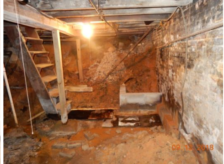
Basement - active water intrusion
