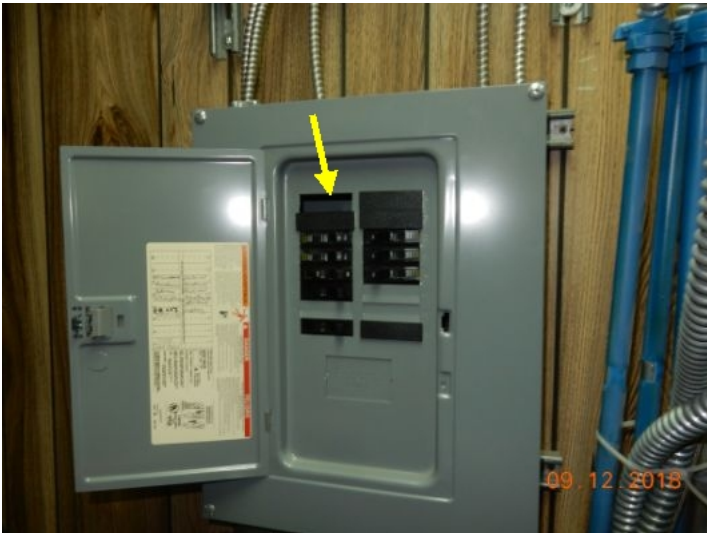
Open knockouts panel enclosure, electrocution hazard, install proper filler plates. - 2nd floor
