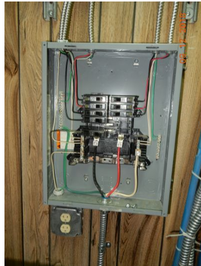
Electrical panel interior - 2nd floor
