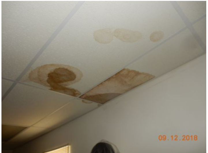
Wall/ceiling moisture stains, tested as 100% moisture content. 2nd floor ceiling Have licensed contractor evaluate/repair.
