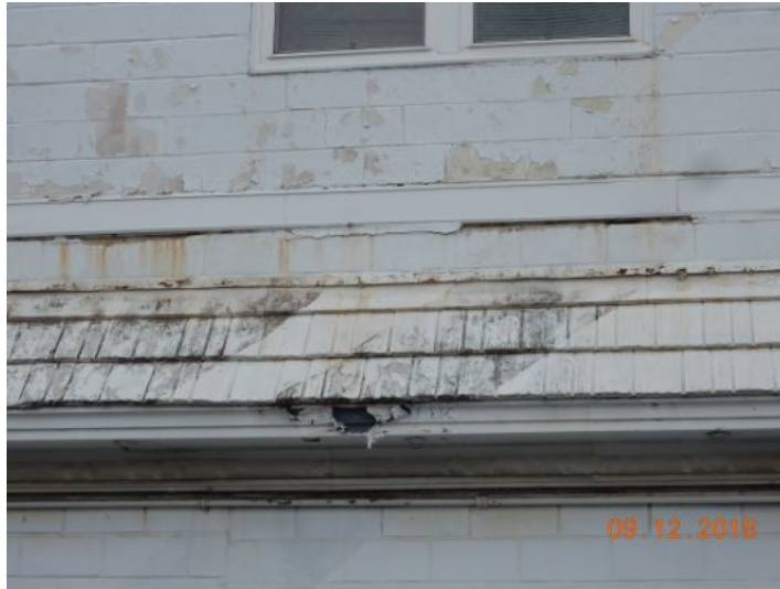
Front mansard roof may be leaking to interior
