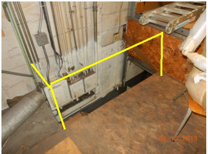
Recommend installation of guard railing at loft opening dropoff.
