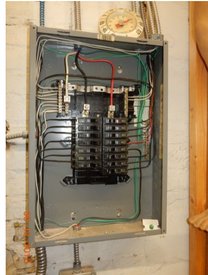
Electrical panel interior -shop/warehouse
