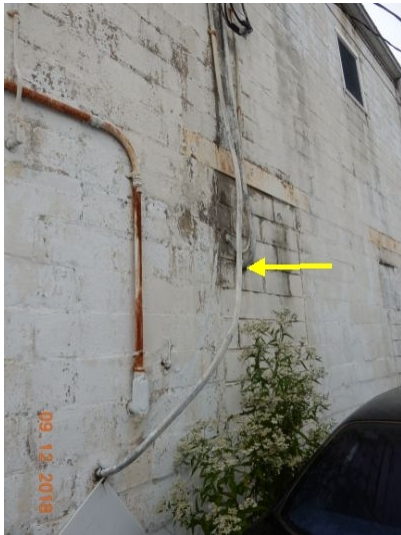
Secure loose service entrance cable to side wall.
