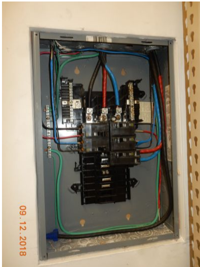
Electrical panel interior -shop/warehouse
