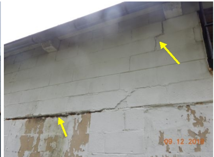
Some settlement cracking at concrete block walls, various locations. Cracks are fairly typical for an older masonry structure. Recommend sealing cracks and monitoring.
