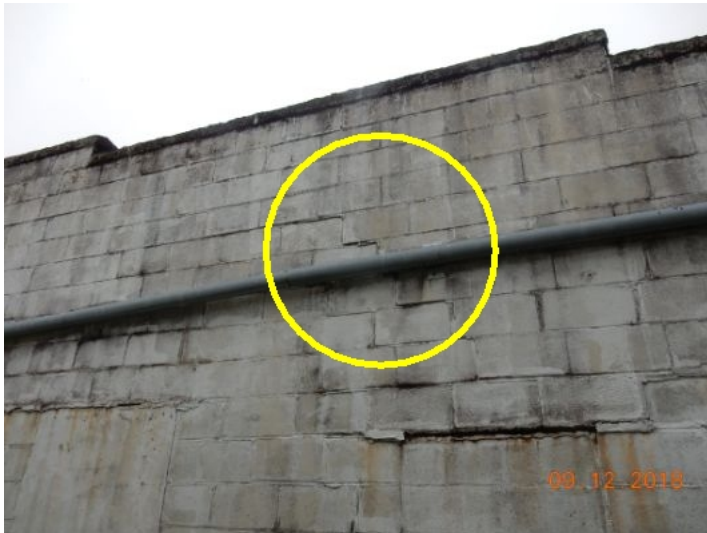
Some settlement cracking at concrete block walls, various locations. Cracks are fairly typical for an older masonry structure. Recommend sealing cracks and monitoring.
