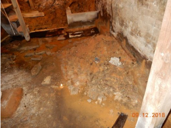
Water pooling in basement
