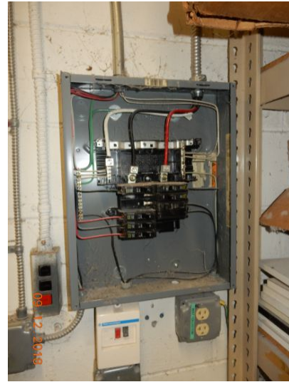
Electrical panel interior - shop/warehouse
