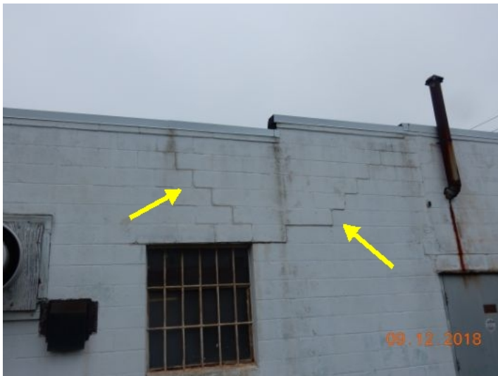
Some settlement cracking at concrete block walls, various locations. Cracks are fairly typical for an older masonry structure. Recommend sealing cracks and monitoring.
