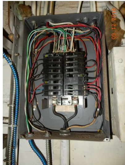
Electrical panel interior
