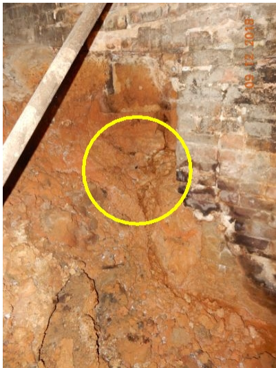
Active water intrusion noted, unknown source.
