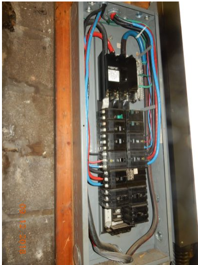
Electrical panel, main office
