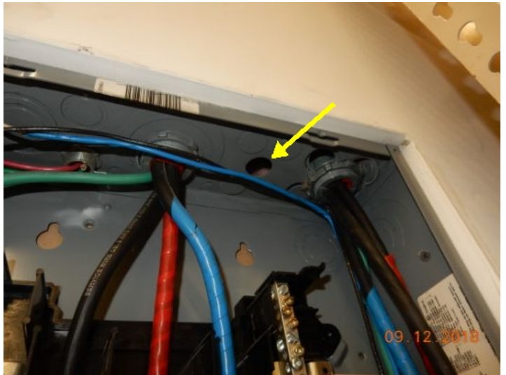
Knockouts need snap-in caps inside panel box. Should be installed to keep mice out of panel box and to avoid potential electrocution hazard. Mold room
