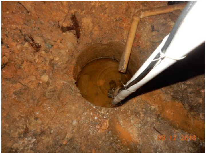
Recommend installing heavy duty sump pump with backup battery
