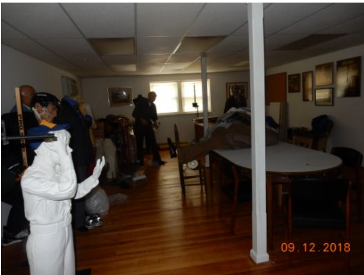
Room with ceiling leak
