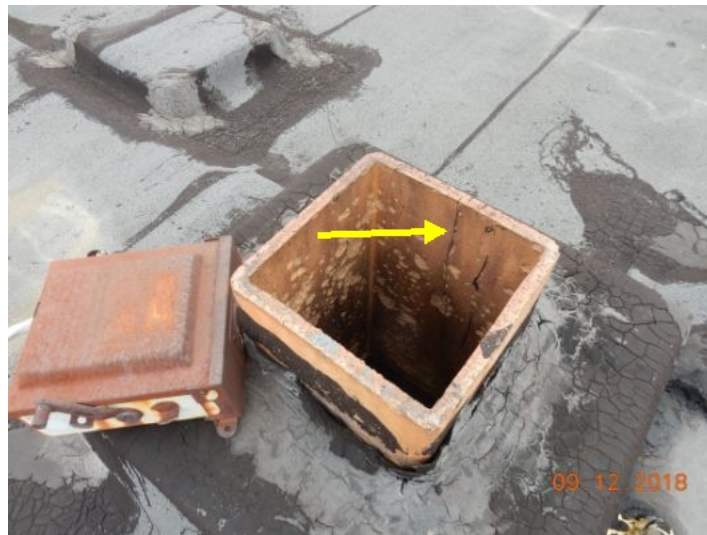
Chimney flue is cracked.
