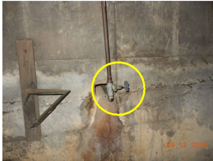
Main water valve location
