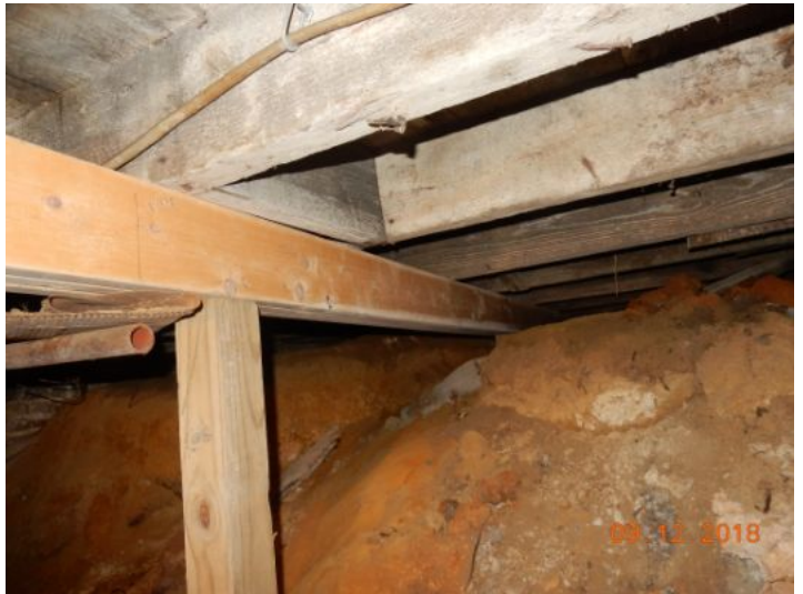
Framing and soil in close proximity, can lead to framing damage
