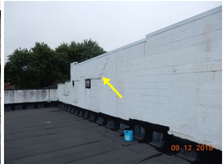
Some settlement cracking at concrete block walls, various locations. Cracks are fairly typical for an older masonry structure. Recommend sealing cracks and monitoring.
