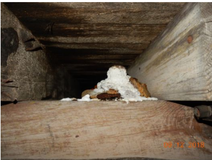
Possible asbestos, recommend testing.
