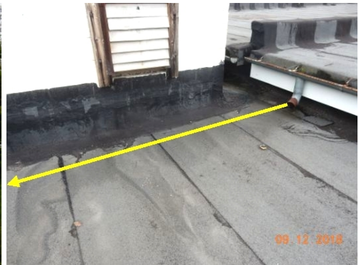
Recommend directing roof downspouts to gutter below
