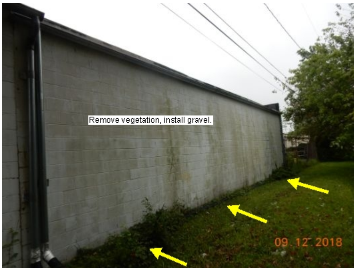
Improve grading as necessary to drain water away from structure
