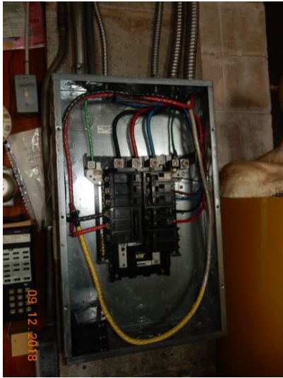
Electrical panel interior- shop
