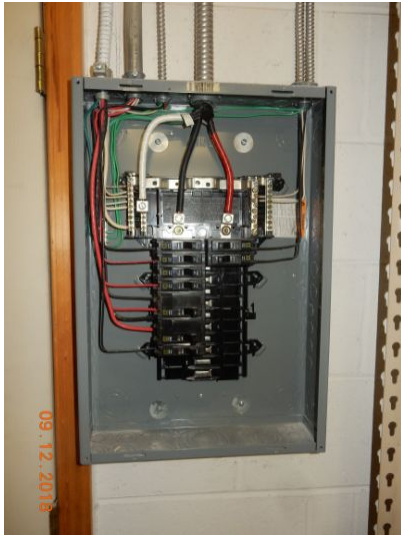
Electrical panel interior- shop/warehouse
