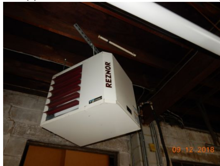
Ceiling mounted gas heaters functional
