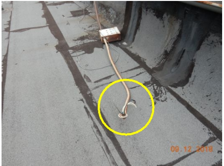
Exposed live wiring at 2 roof locations. Electrocutation hazard. Have licensed electrician remove abandoned wiring. See photos.
