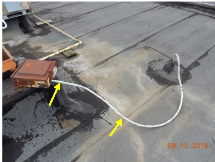
Exposed live wiring at 2 roof locations. Electrocutation hazard. Have licensed electrician remove abandoned wiring.
