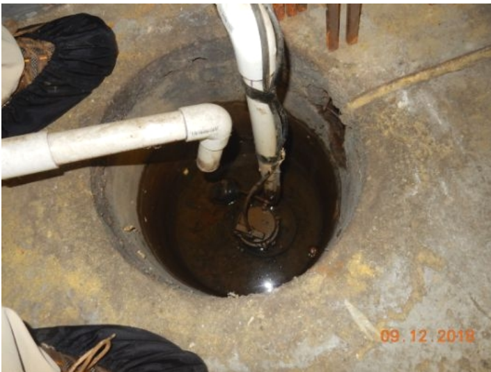
Sump pump float not operating consistently.
