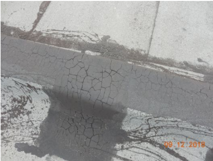
Asphalt cracked, recommend sealing
