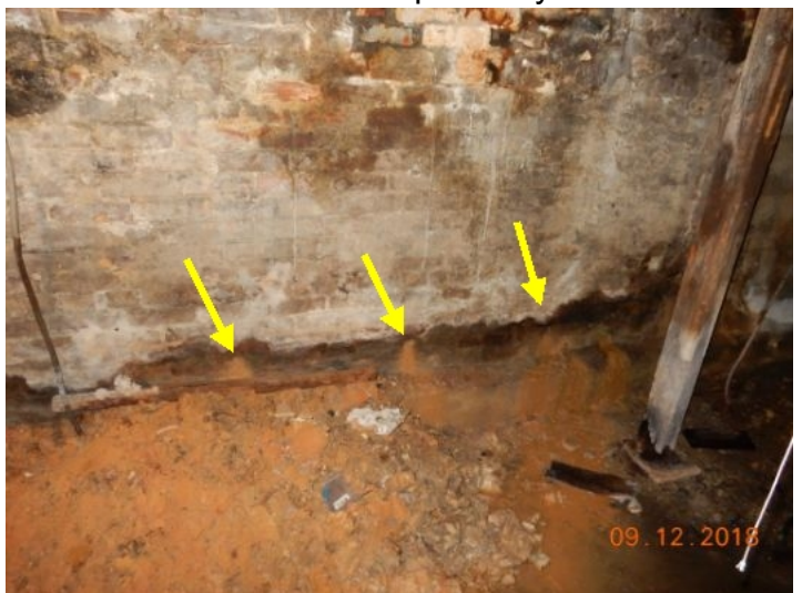
Water intrusion points, source unknown
