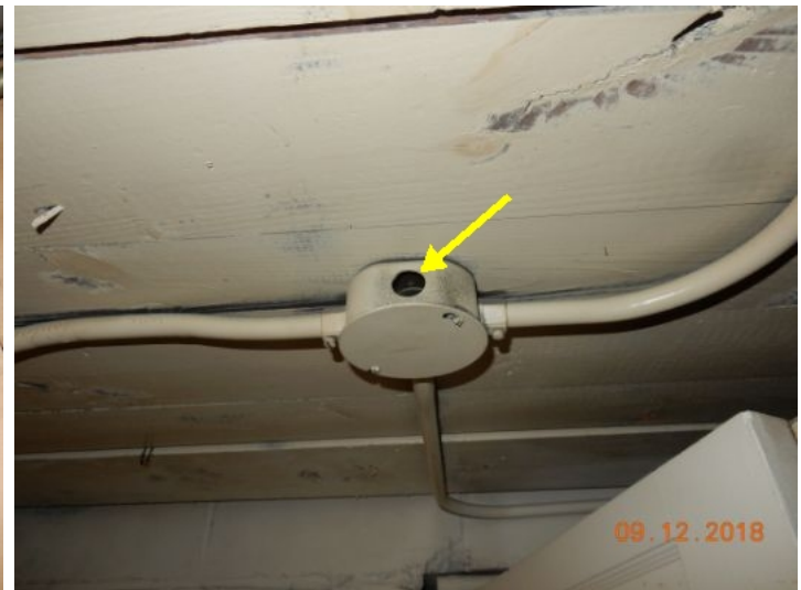
Open knockouts in numerous electrical boxes throughout property.
