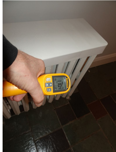
Radiators heated in response to boiler operation.
