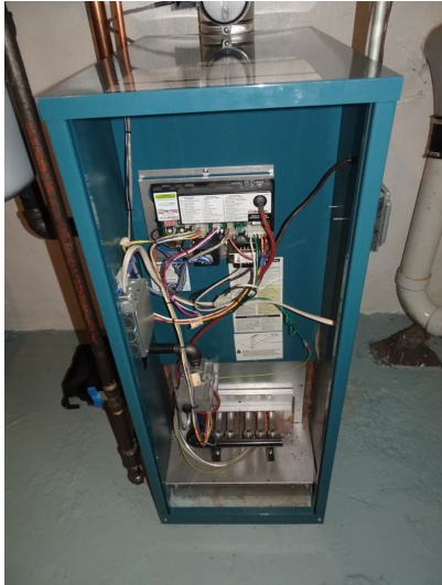
Boiler mfg. date(s) - 2018
