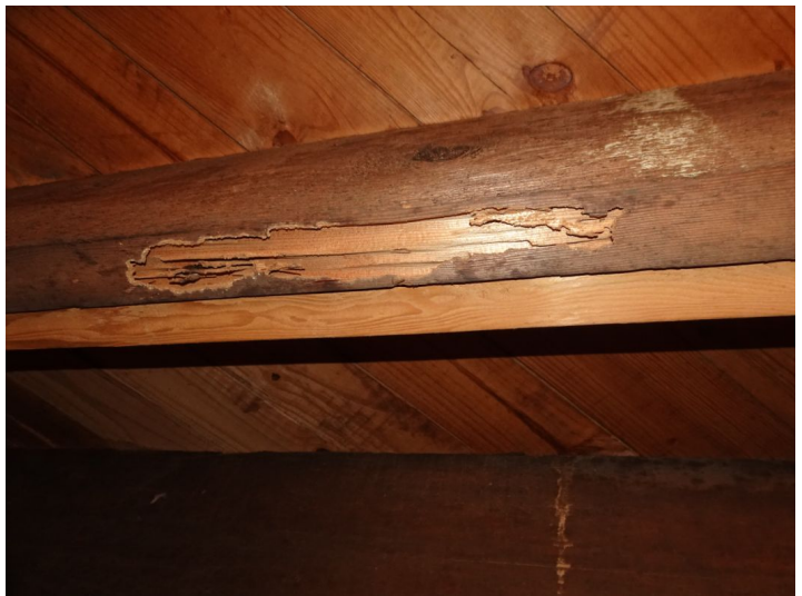
Some basement framing has been altered/reinforced, due to apparent insect damage. You may wish to have a licensed professional evaluate further.
