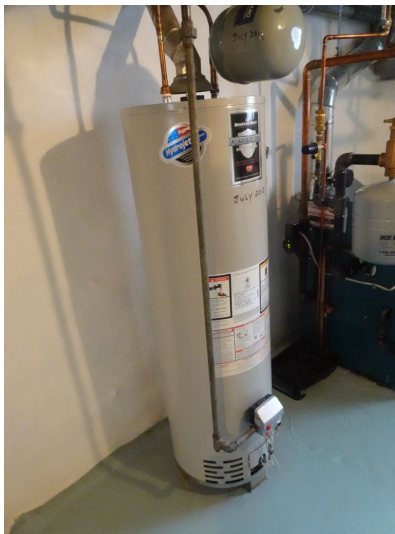
Water heater mfg. date(s) - 2012
