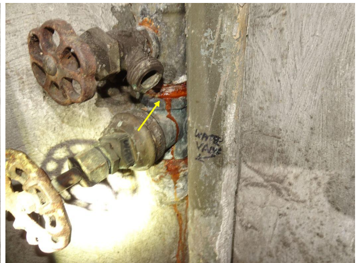
Main water line is leaking near main water valve. Have licensed plumber repair/replace as necessary.
