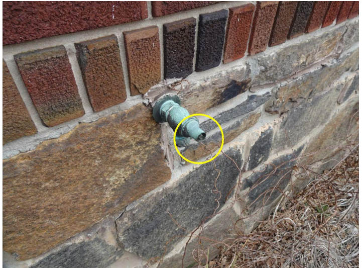
Missing handle at hose faucet, exterior
