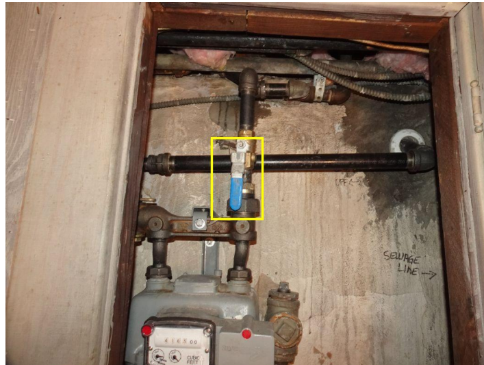
Gas Valve location - front wall of basement in closet
