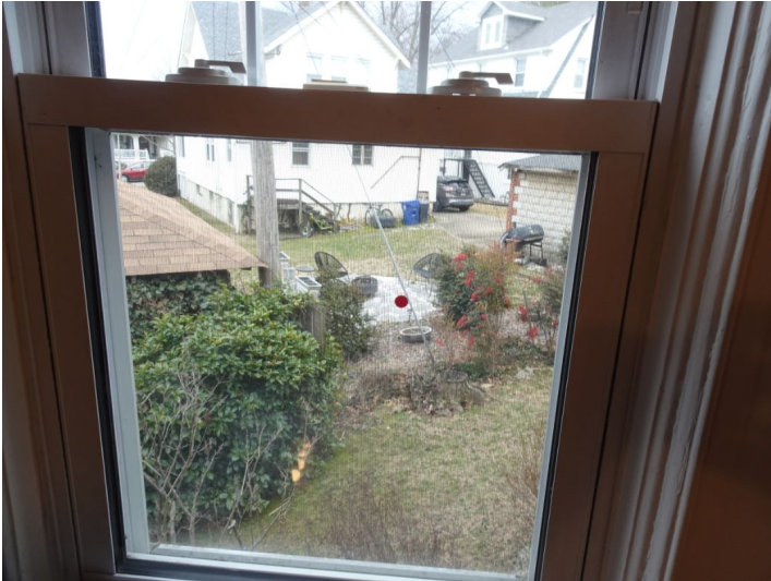
Window sash will not stay open, failed spring balances. Repair. Marked with red dot, kitchen
