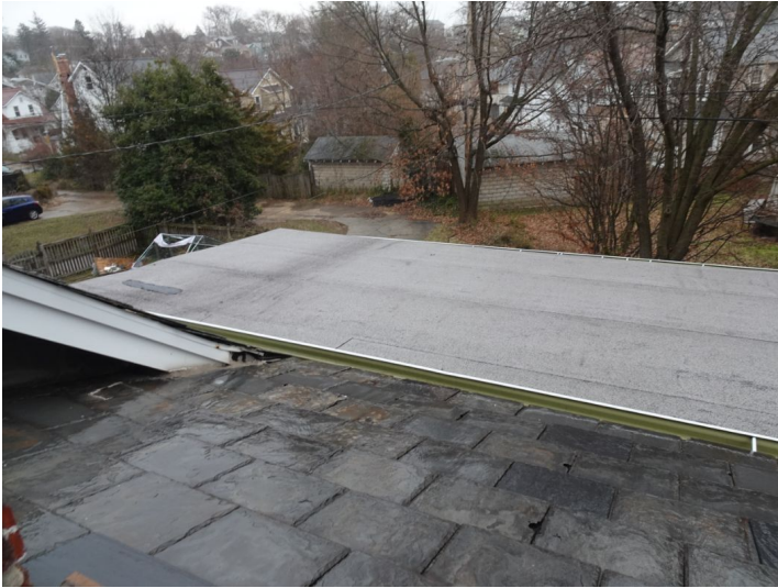
Granulated rubber roofing in older, worn condition, recommend coating with white roofing compound or replacing.
