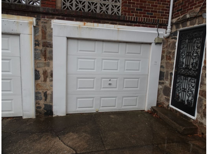
Note: Right garage was locked, could not inspect. Have it inspected before final walkthrough.
