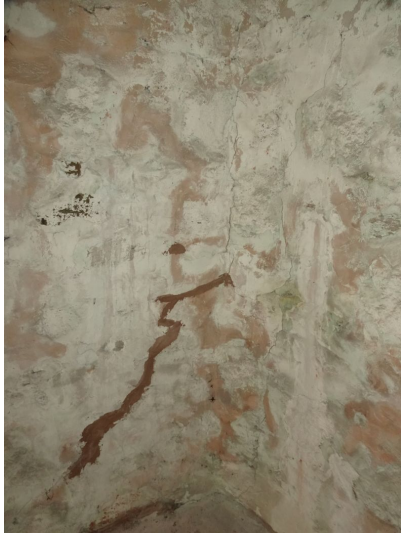
Minor settlement cracks in garage walls. Recommend sealing and monitoring.
