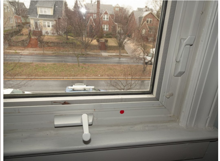
Casement window on 3rd floor will not open. Repair as necessary
