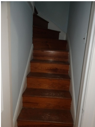
Hand Rail Components missing at attic stairs. Install to promote safety.
