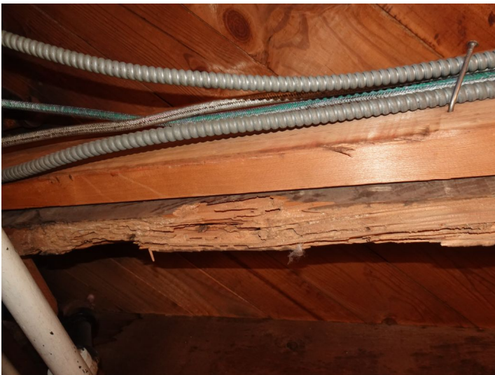
Some basement framing has been altered/reinforced, due to apparent insect damage. You may wish to have a licensed professional evaluate further.
