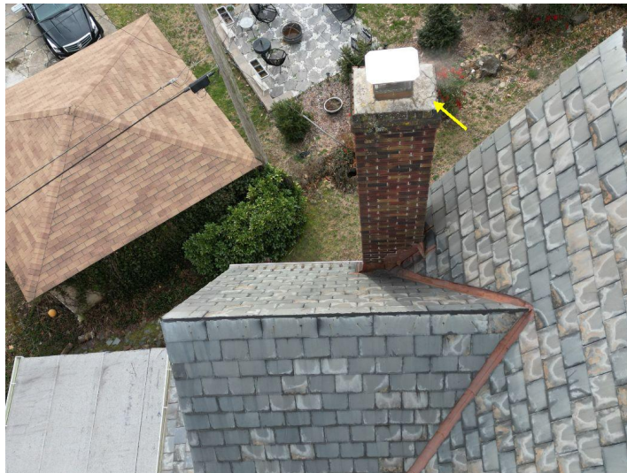
Cracks in concrete chimney crown. Repair as necessary
