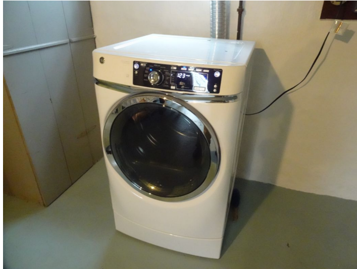
Washing machine and dryer operational
