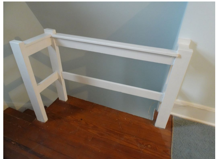
Openings at attic stairs exceeds 4 inch spacing, which is not considered safe by today's standards. Adjust to promote safety.
