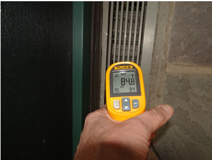
Heat output at vent
