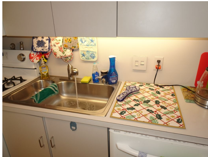
Non GFCI protected outlets near sinks in kitchens, 1st and 2nd floors, recommend replacement with GFCI type to promote safety.
