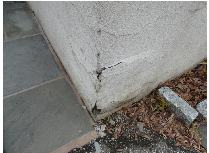
Minor damage to stucco siding. Repair as necessary.
