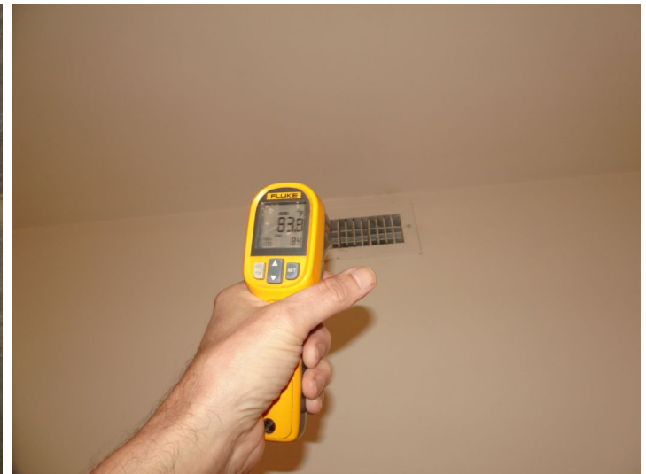
Heat output at vent
