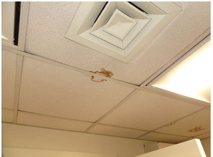
Apparent wall/ceiling moisture stains, tested as normal moisture content at time of inspection.
