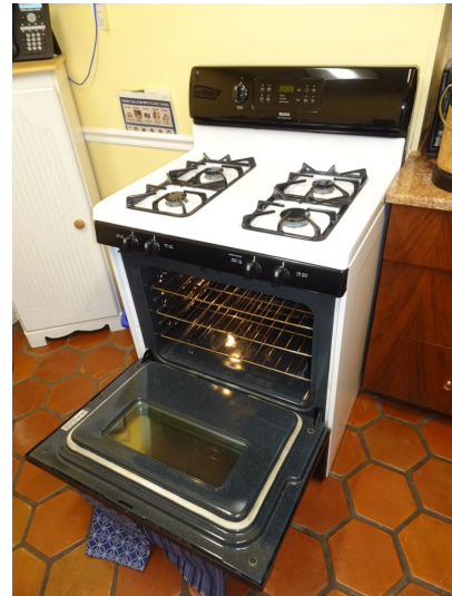
Stove anti tip bracket not installed, all stoves, 1st and 2nd floors. Anti tip brackets are required to be shipped with every unit. It is a safety device intended to prevent the stove from tipping over if a person falls on the open oven door. Install to promote safety.
