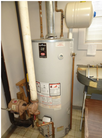
Water heater mfg. date(s) - 2014
