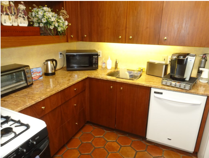
Non GFCI protected outlets near sinks in kitchens, 1st and 2nd floors, recommend replacement with GFCI type to promote safety.
