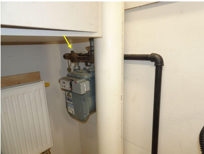
Gas Valve location - Rear utility room
