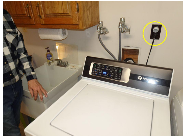
Non GFCI outlets near laundry sink, recommend converting to promote safety.
