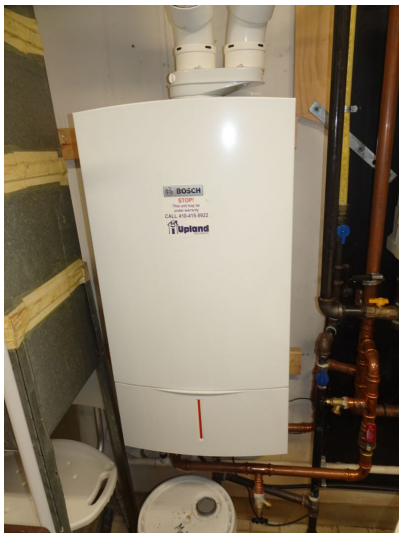
Boiler mfg. date(s) - C. 2018
