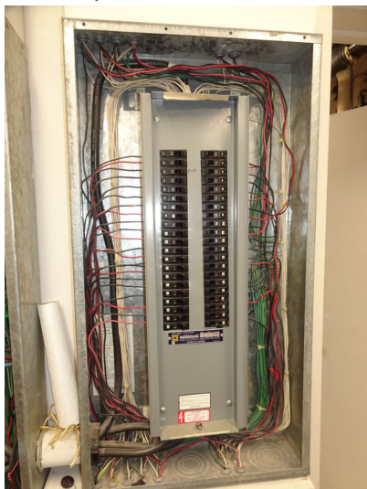
Panel Utility room
