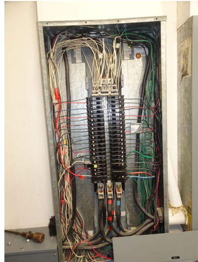
Panel Utility room
