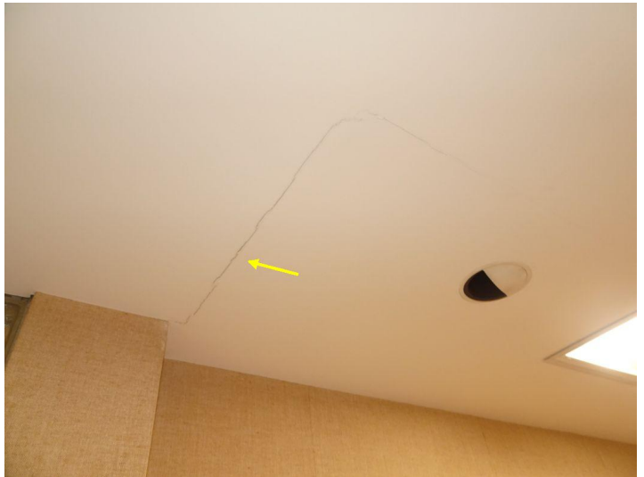
Minor settlement cracks and nail pops noted, which is normal for a property of this age.
