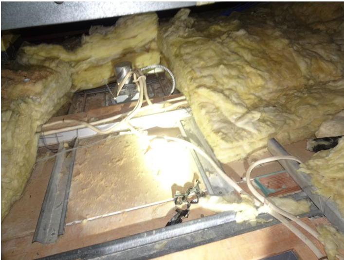
Fiberglass Insulation is installed haphazardly, missing in some areas.
