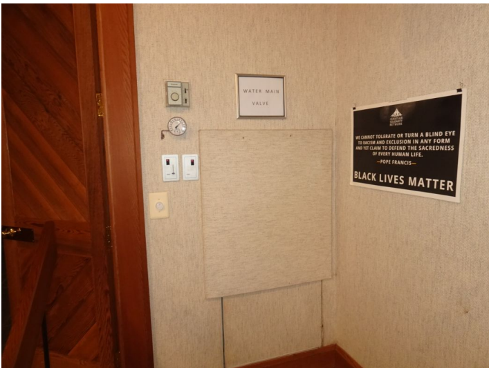
Main water valve location - Auditorium front of bldg. in access panel
