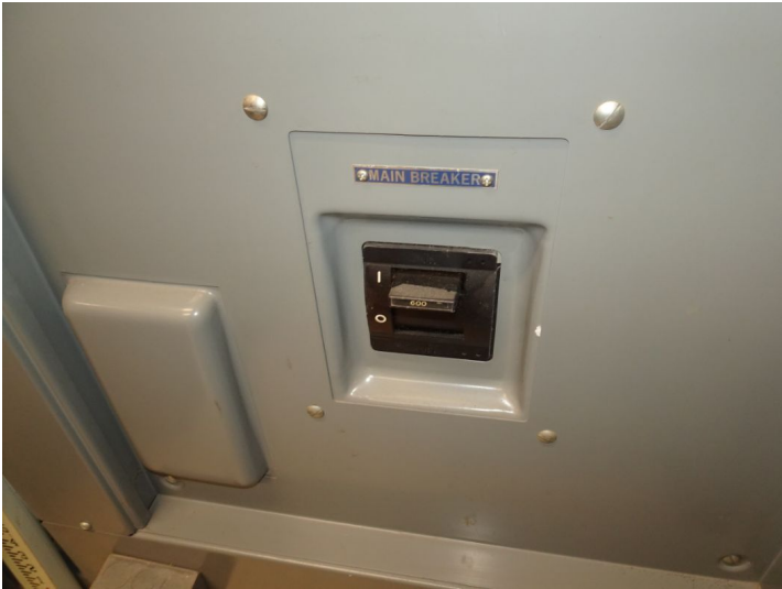
600 amp main breaker switch
