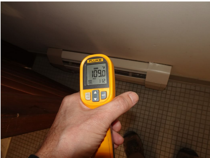
Baseboard heaters operational
