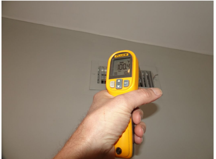
Heat output at vent
