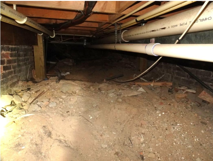
Crawlspace vapor barrier is missing. Recommend installing 6 mil polyethylene sheeting.
