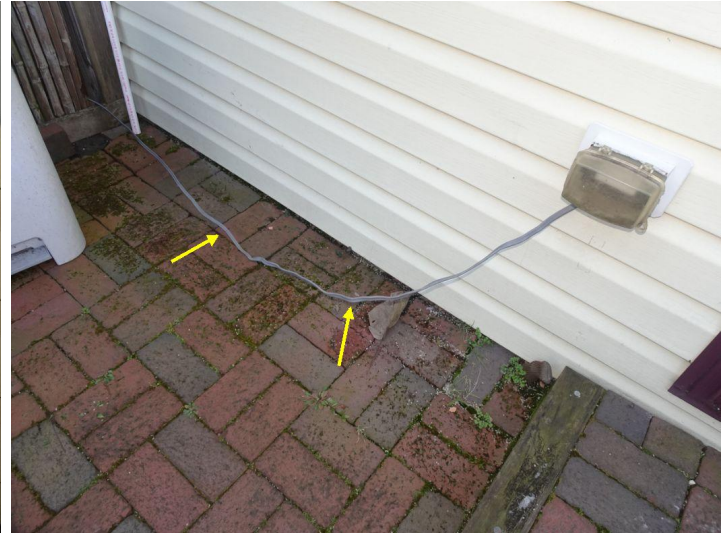
Wiring from outlet to light fixture at parking pad is not professionally installed. Wiring is loose. Secure as necessary.
