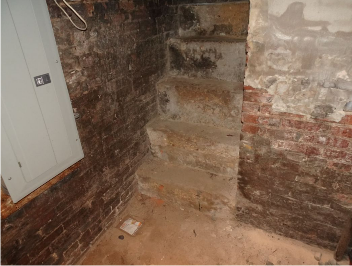
Hand Rail Components missing at basement stairs. Install to promote safety.
