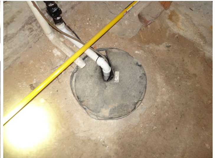
Sump pump operational
