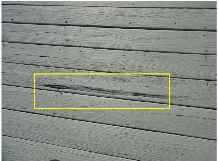
Replace rotted deck components as necessary
