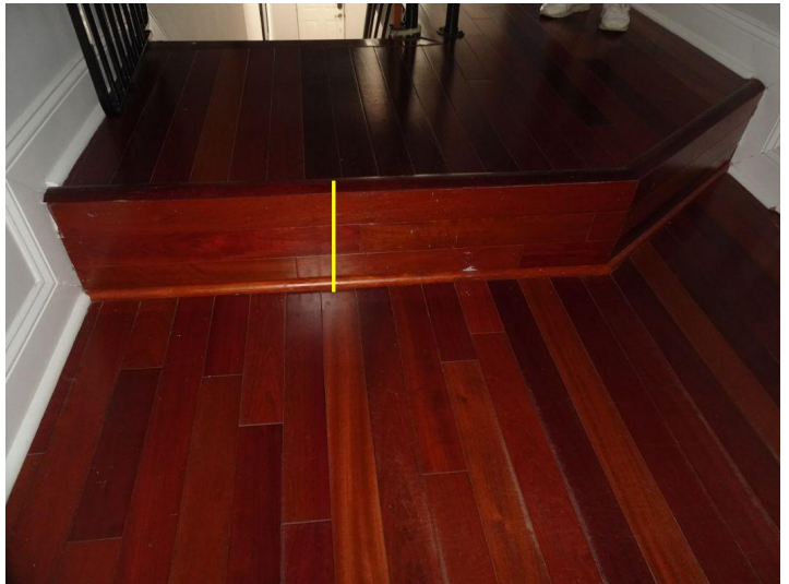
Overheight step 2nd floor. Use caution
