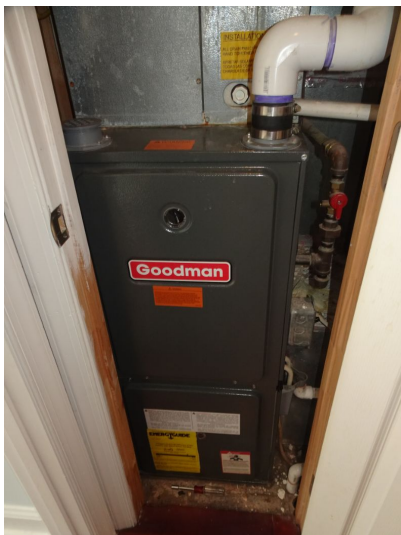
HVAC unit mfg. date(s) - 2004 - 2nd floor
