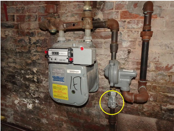
Gas Valve location - Front wall of basement
