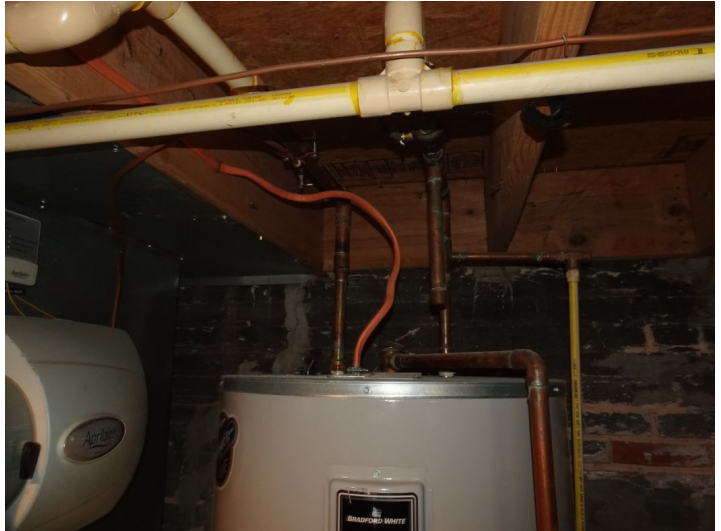
Expansion tank not installed. An expansion tank is required to be installed on all plumbing systems having a pressure regulator or check valve or on new installations.
