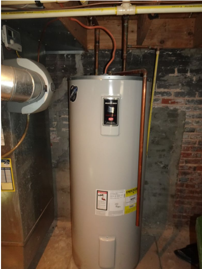
Water heater mfg. date(s) - 2012
