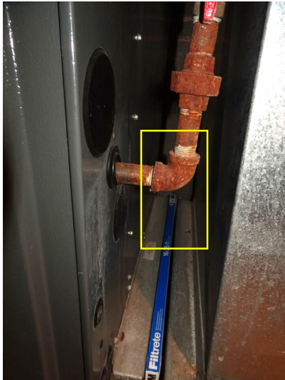
Sediment trap not installed on gas supply line to hvac unit in basement. Install.
