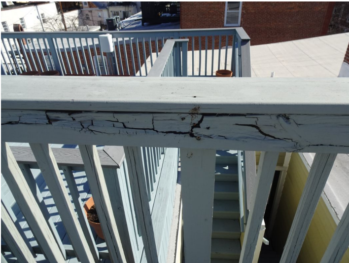
Replace rotted deck components as necessary
