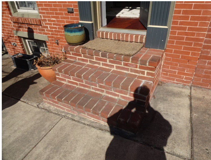
Recommend installation of hand railing at front steps to promote safety.
