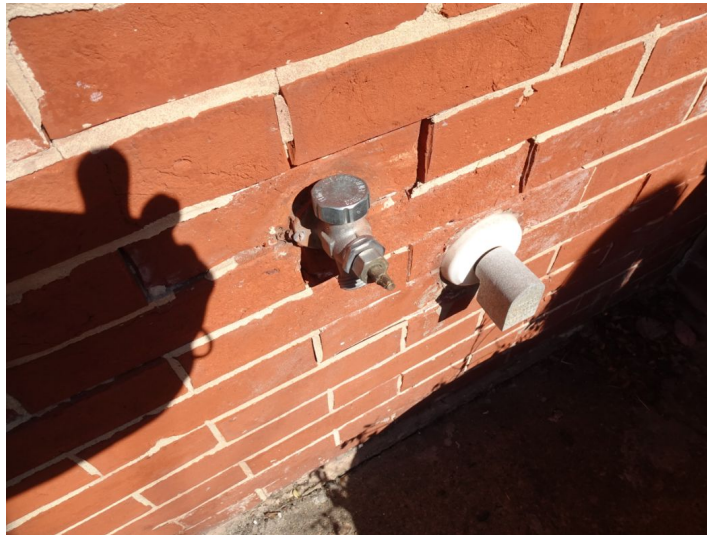
Handle missing at front hose faucet. Install.
