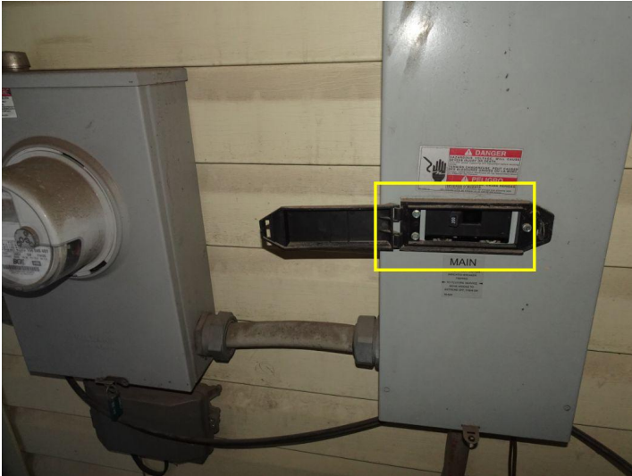
Main electrical shut off switch. Above entrance to basement
